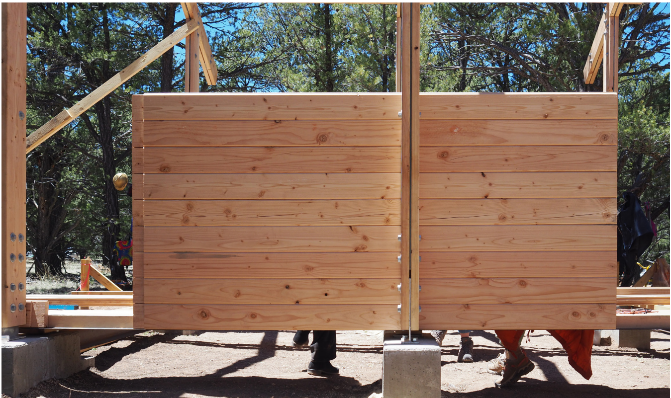
Figure 6. Detail of the cantilevered SLT floor and wall assembly during construction. Image credit CU Denver
