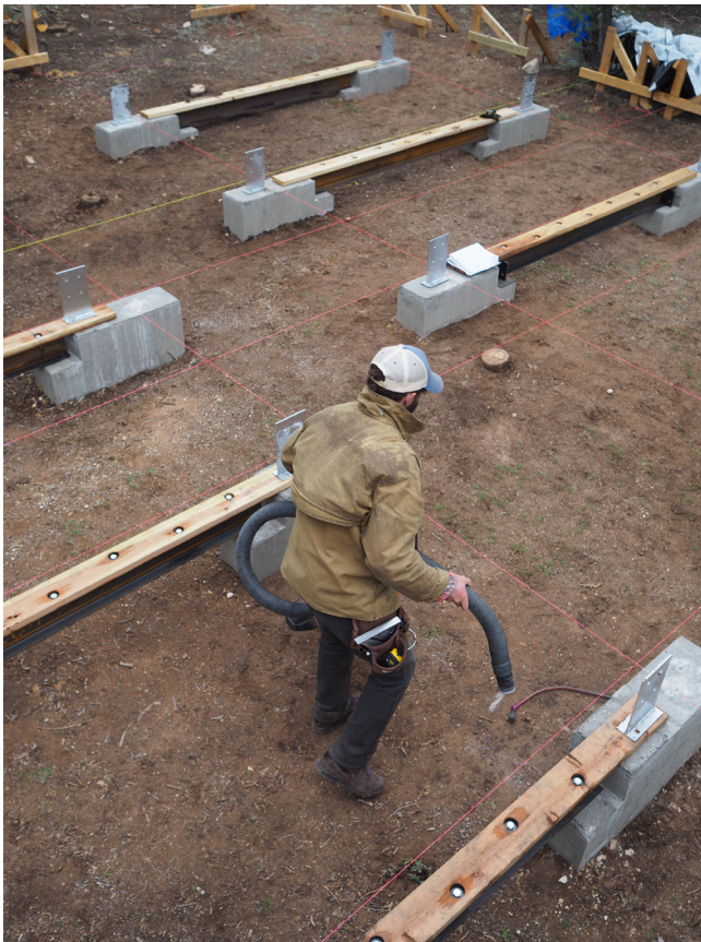
Figure 7. The foundation points and beams required to support two of the cabins. Image credit Rick Sommerfeld
